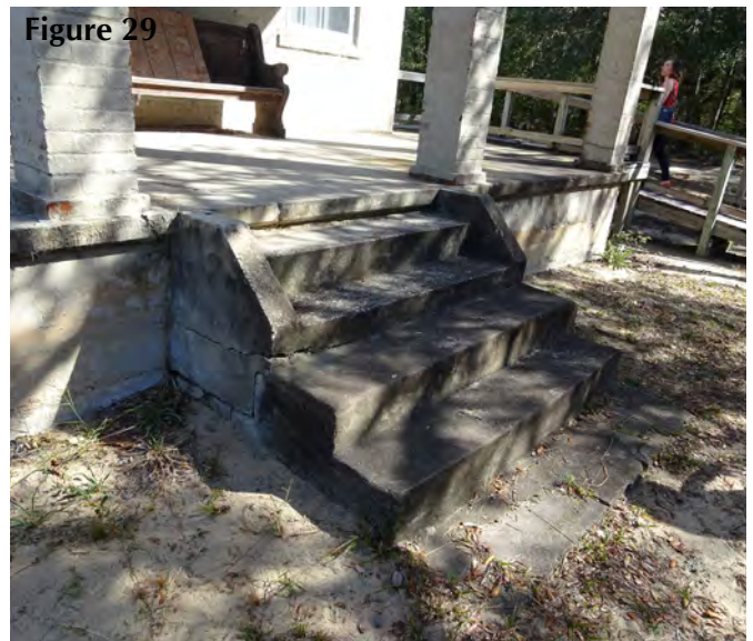
Stairs Notice differential riser heights
