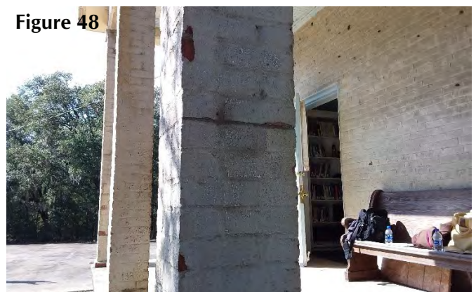
Figure 48 Crack in masonry porch column
