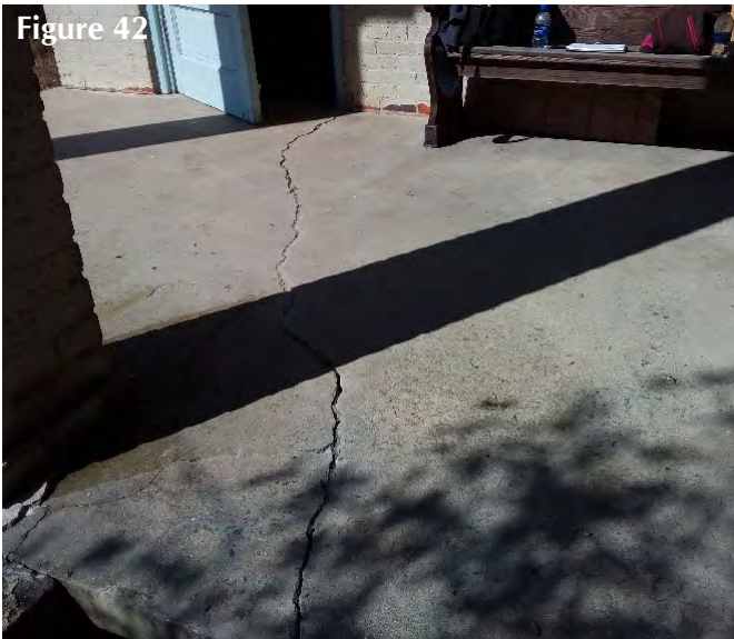
Large crack in front porch slab
