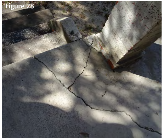
The porch floor slab has cracked. October 2017
