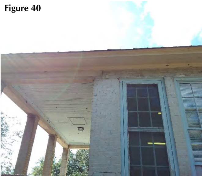
Stairstep cracking in masonry wall with brick out-of-plane
