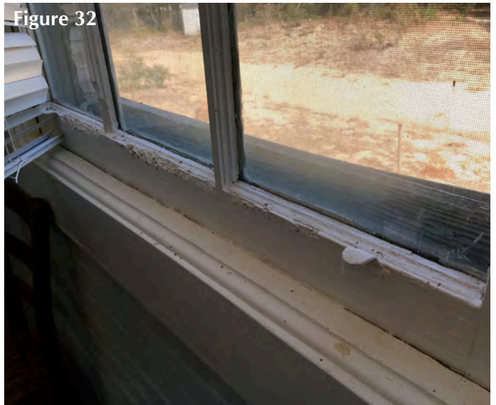
Damage to interior window sash
