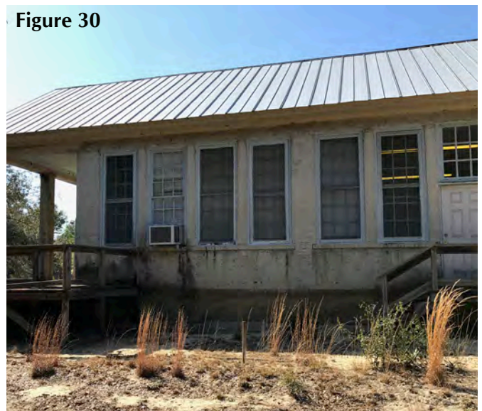
East Elevation- Staining form excess water on the east wall
