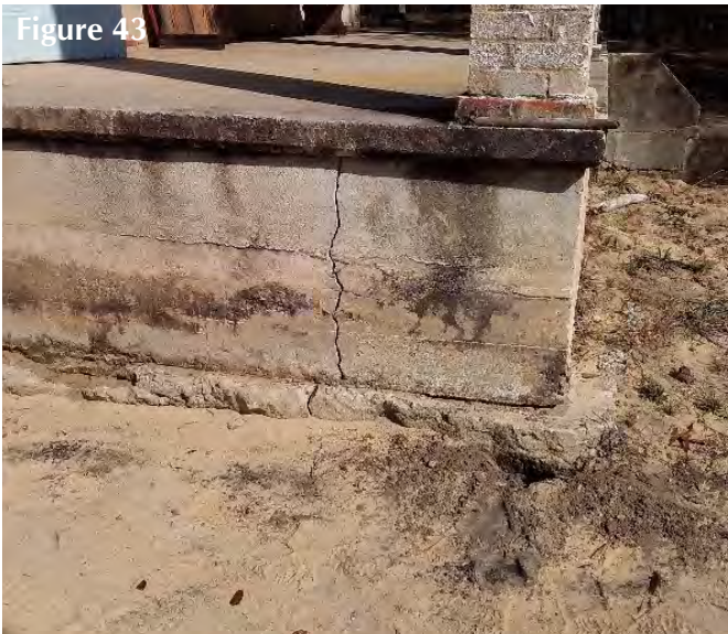
Crack in foundation wall at SW corner and grade eroding
