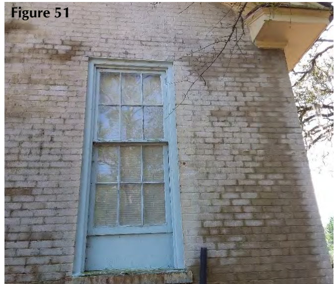
Deflected steel lintel at rear (North) wall
