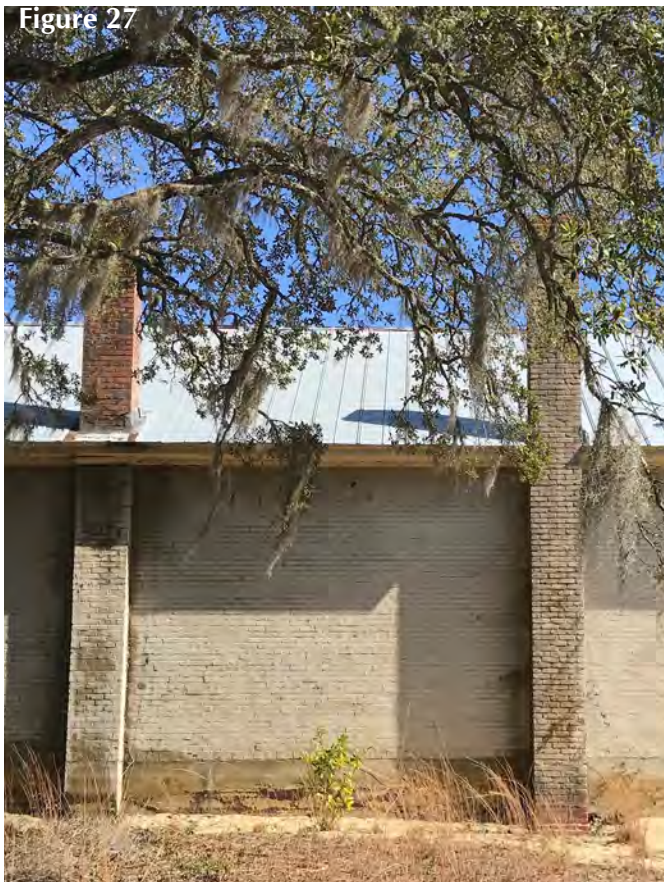
Figure 27 The chimneys on the west elevation. Note water staining around the north chimney.
