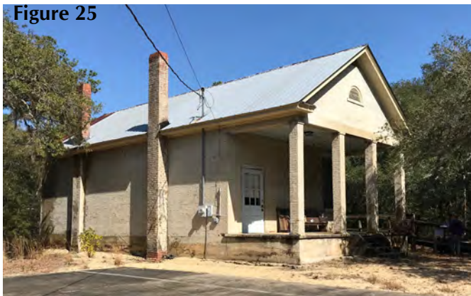
Figure 25 Erosion at southwest corner
