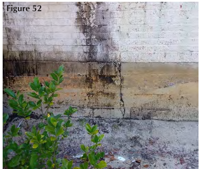
Foundation wall crack along eastern elevation
