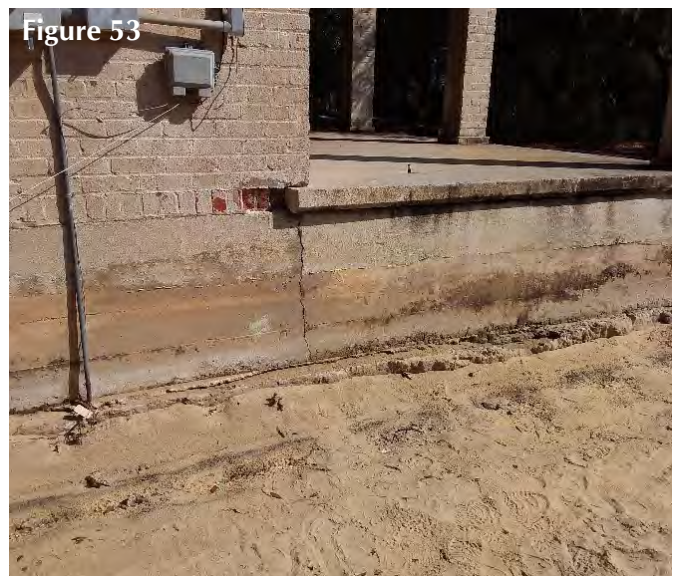
Crack in foundation wall and loose brick SW corner
