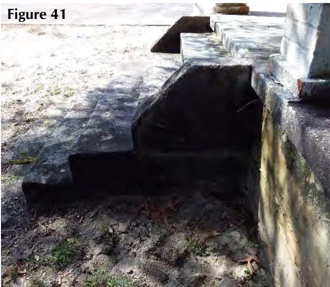
Grade eroding from stair at front of building
